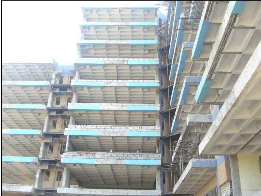
Fig.11 View of the building after strengthening of beams by using FRP Wrapping. It is visible on the beams as blue color.
